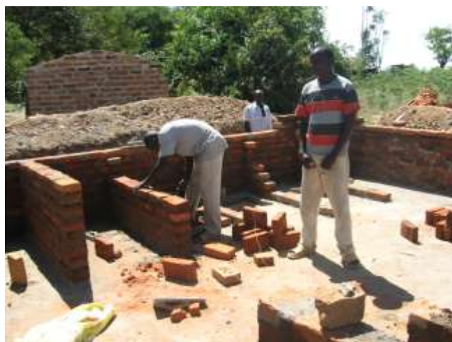
Picture 7: The new VIP latrine under construction at the Mbalibali Primary School.
