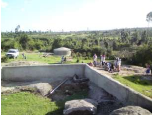
Picture 4: Rock catchment with water storage tank downhill
