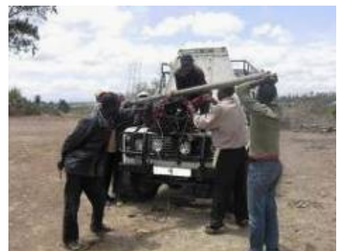
Picture 7: Seven men helping us lift the engine block out of our Land Rover in our front yard
