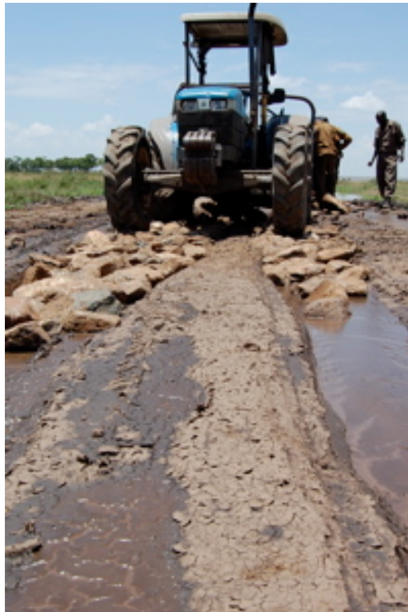
Heavy rain destroyed a section of river road. The road team repairs the road following the storm
